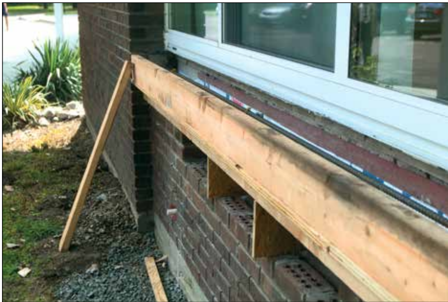
Photos by Joseph Cole Above: The new gymnasium floor at Peck Place was itself a $100,000 project according to Orange Board of Education Facilities Administrator Mike Luzzi. Right: New concrete windowsills needed to be poured at the school in order to do away with potential PCB contamination. Story Inset: Contractor employees work in the final weeks before classes are scheduled to start to put the school's stage together.
